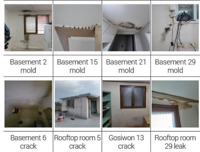
Figure 1. Cases of inadequate structure safety
