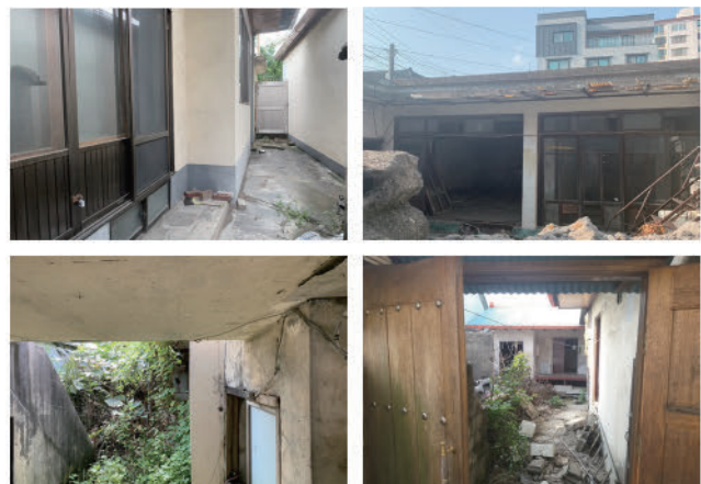
Figure 6. Status of vacant houses in residential areas
